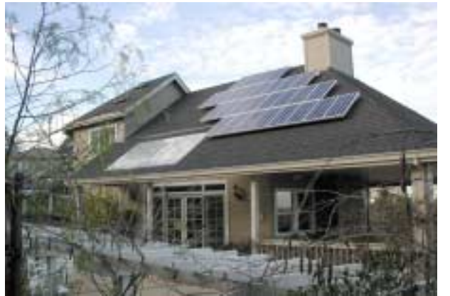
2.0 kW AC Grid-connected, net metered, battery back-up
