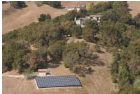
31 kW AC Grid-connected, net metered battery back-up
