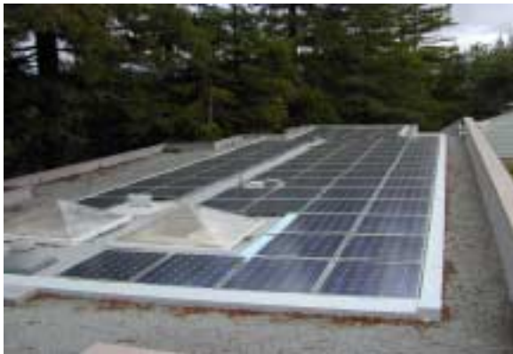
9.8 kW AC PowerGuard thermally insulating solar electric roof tiles. Grid-connected, net metered, battery back-up
